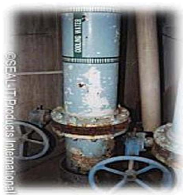
Fig. 3. Crevice Corrosion in a Flange
