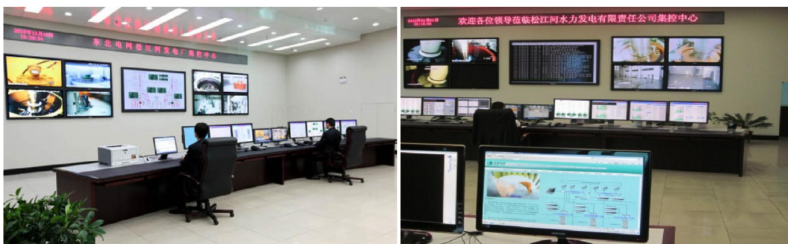
Fig. 13. online monitoring and condition-based DSS information platform of Songjianghe Hydropower Plant
