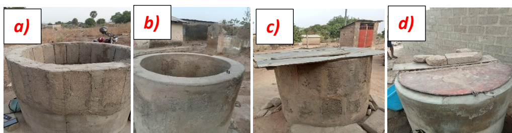
Fig. 2. Open and closed wells in the Camp-Adagbe (a, b) and Tibona (c, d) districts
