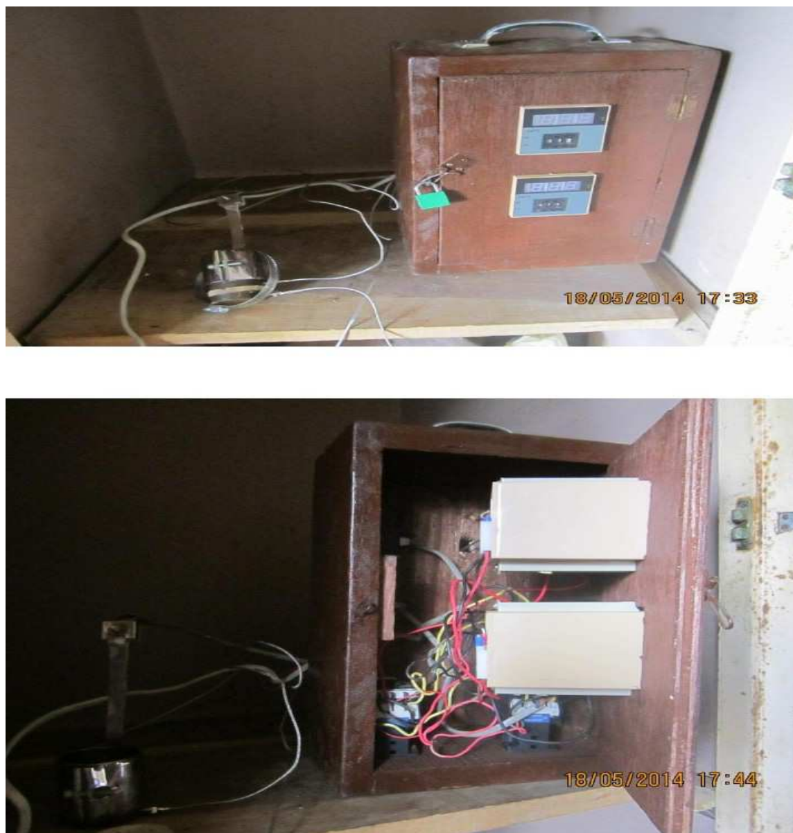
Fig 5 The front and inner components of the Electrical set-up
