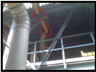
Fig 4: Points of heavy vibration (on-site location)
