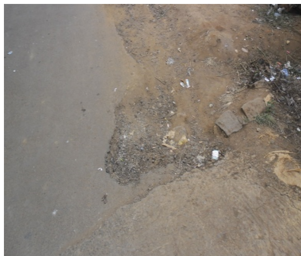
Fig. 2. Damaged road surface in Periyarnagar
