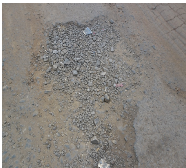
Fig. 3. Damaged road surface in Agalar
