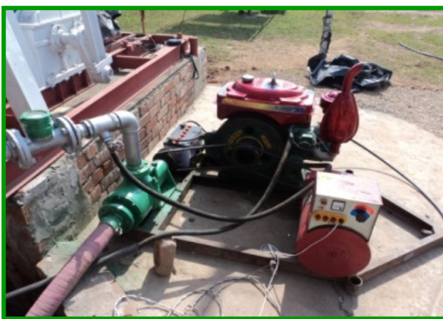
Fig. 2 Dual-fuel Pumping system Installed at NARC, Pakistan
