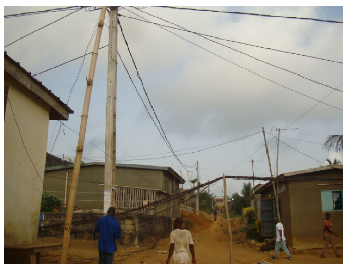
Figure 3: anarchic connections of electric cables
