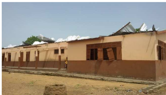
Figure 1: Damages to a school building by the 10/05/2016 rainstorm in Bongo
